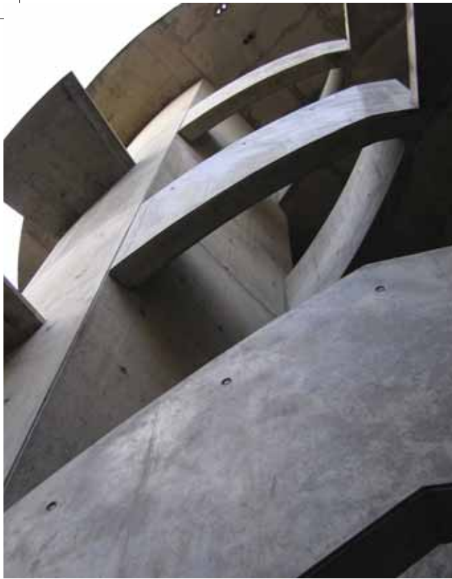
Above Lift shaft, balustrade beam and half-landings of the drum stair before the precast treads were fixed
